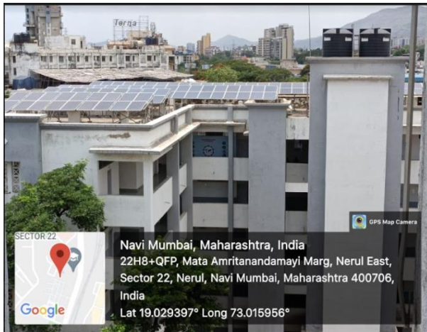
Fig. Solar roof on TEC Building
