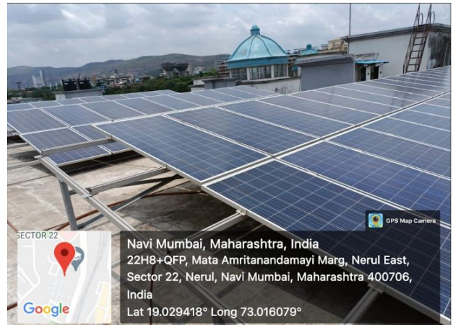
Fig. Close view of solar panels on TEC Building
