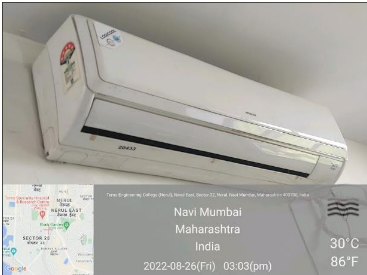
Fig. Power efficient equipment 5 star rated split AC
