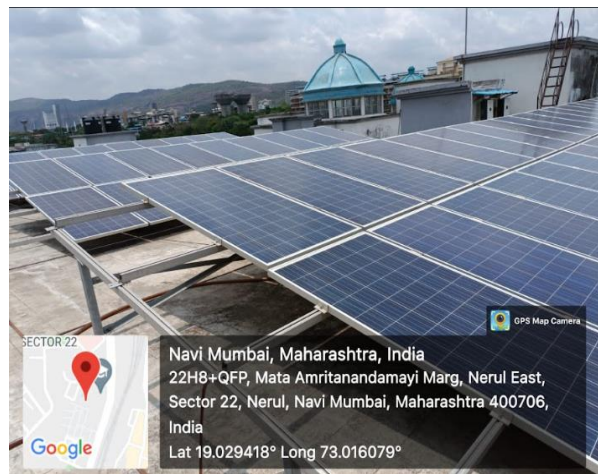
Fig. close view of solar panels on TEC Building
