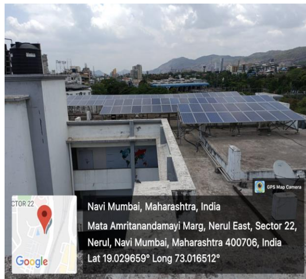
Fig. Solar roof on TEC Building
