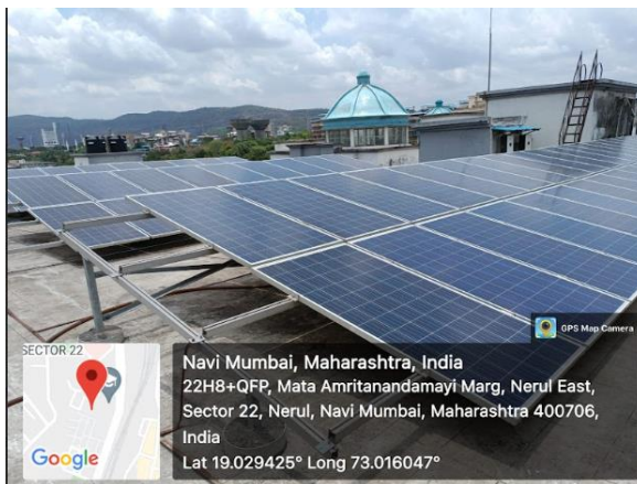
Fig. Solar panel on TEC roof
