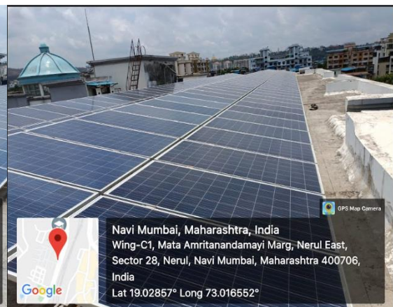
Fig. Clean energy Solar panel on TEC roof
